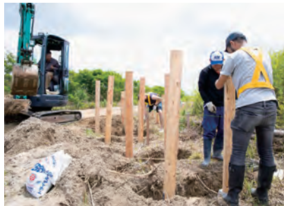
1 まずは木道の土台となる杭を打ち込んでいきます First of all, posts that form the base of the path were driven into the ground.
