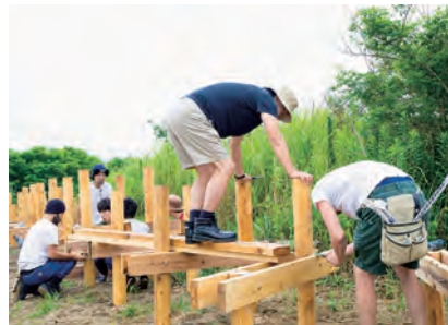
3 ゆるやかな傾斜をつけるため、横板の高さを調整 The height of the beams was adjusted to create a gentle slope.
