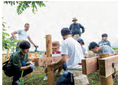
2 土台を補強する横板の打ち込み Horizontal beams to reinforce the base were secured to the posts.
