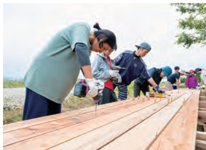
5 床面を参加者総出で固定 The planks were drilled into place by all the participants.
